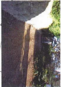
Photo shows the existing surface has worn been worn away by vehicles - surface affected by leaf fall from trees along the route of the path.
